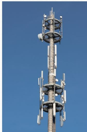
5G Antenna Tower
